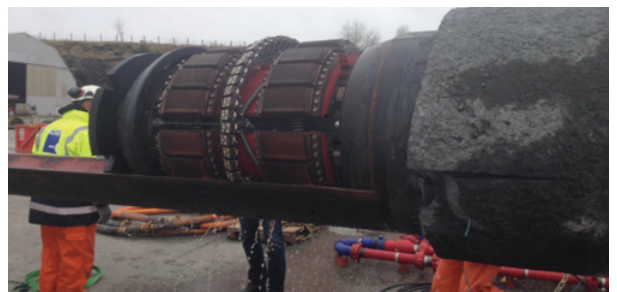
Gjøa: subsea-to-subsea intelligent pigging operation
