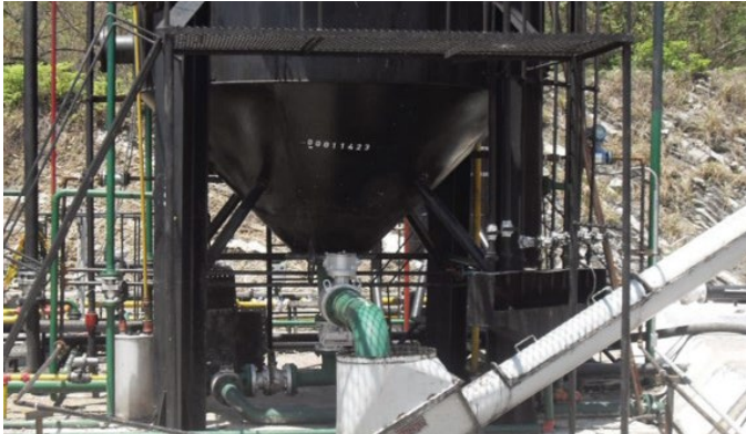
Figure: Heater-treater conical bottom with screw conveyor.
