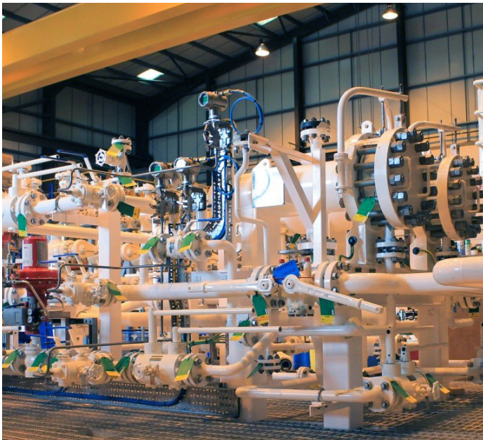
Operator/Project: ConocoPhillips, Alder Solutions Provided: Produced Water Treatment Module Year Delivered: 2014
