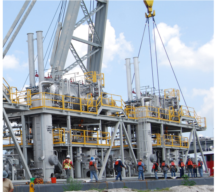
Operator/Project: Noble, Tamar Field Solutions Provided: Glycol Regeneration Packages Year Delivered: 2012
