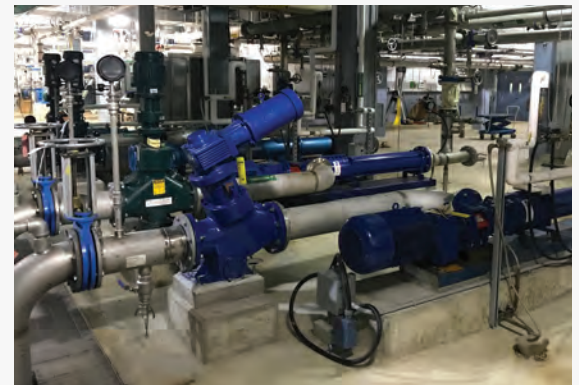
Wastewater treatment plant in Canada. Products shown: EZstrip TR Muncher and EZstrip Progressive Cavity Pump
