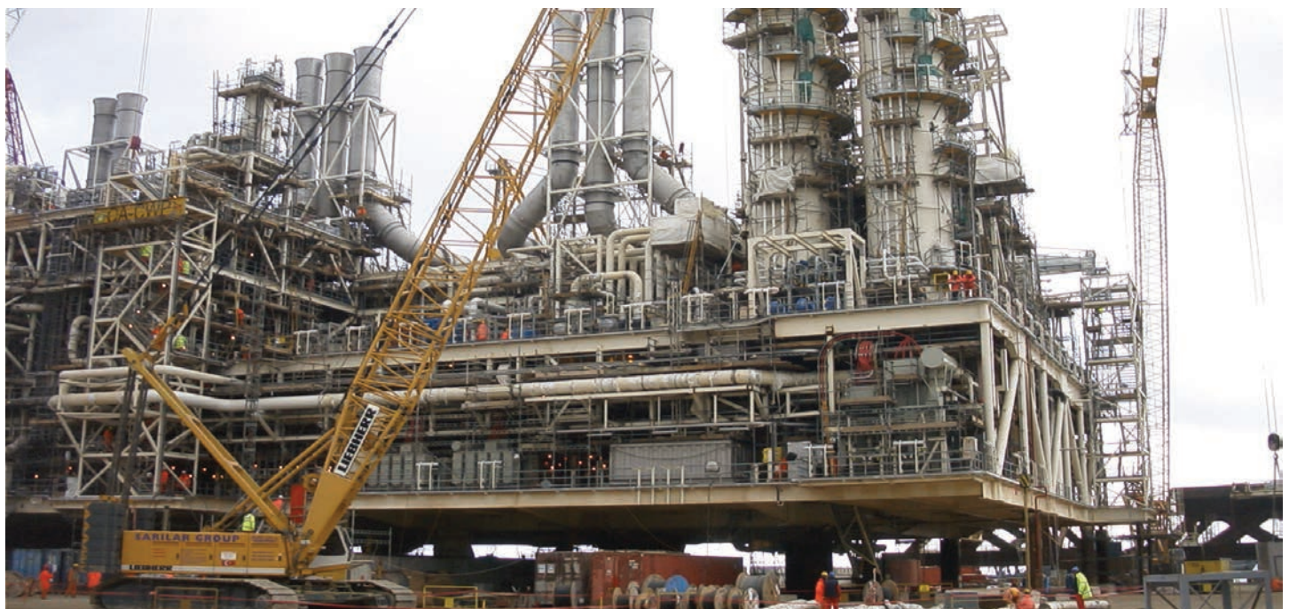
C&WP Platform in Production
