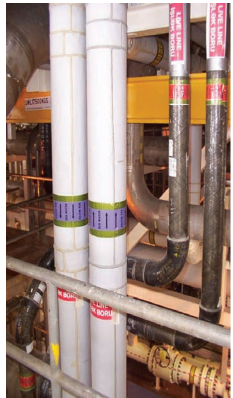
Bondstrand Cooling Water Lines in Service
