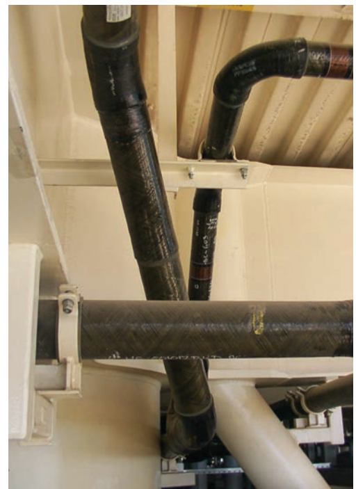
Crossing of Several Pipe Systems
