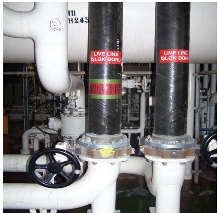
Flanges to Connect to Steel Piping
