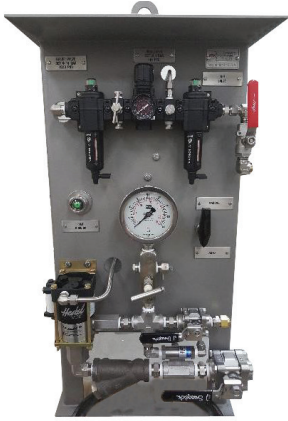
HPU and Valve Control Systems
