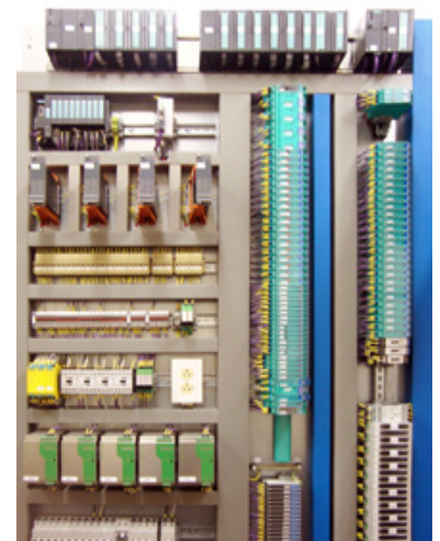
SIMATIC S7 PHM Control Panel
