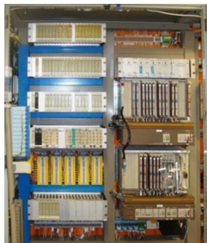
SIMATIC S5 PHM Control Panel
