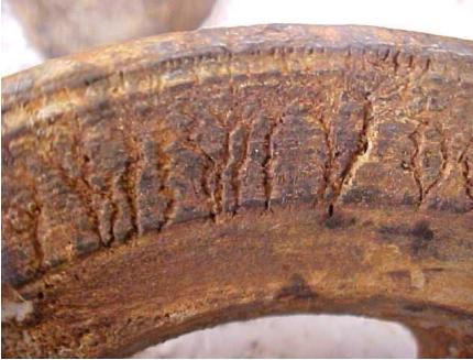
Supreme Seat Corrosion
