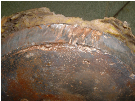
Solids and Corrosion
