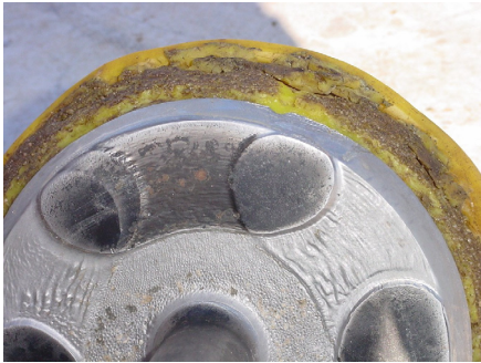
Valve Manually Rotated
