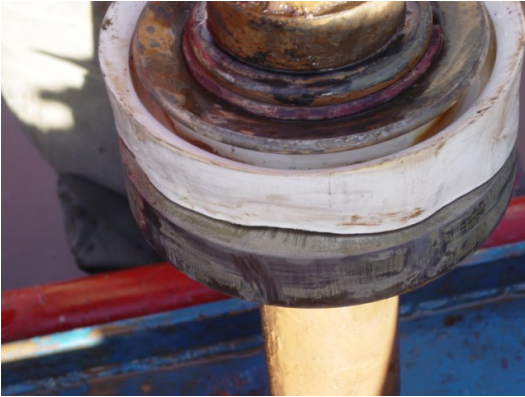
White Lightning Heat Damage
