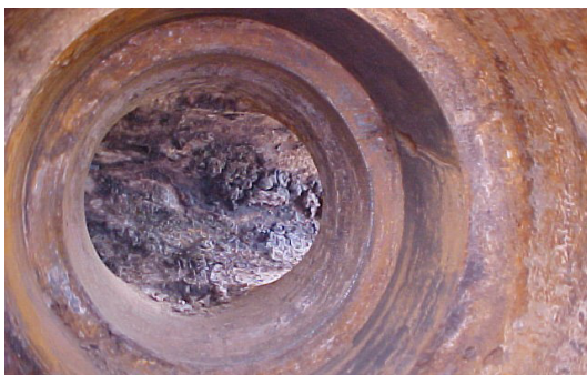
Washed Out Module (Module Worn Out)
