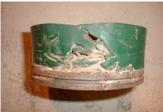
Green Duo Extrusion Damage
