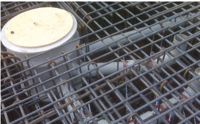
Manholes within raft slab
