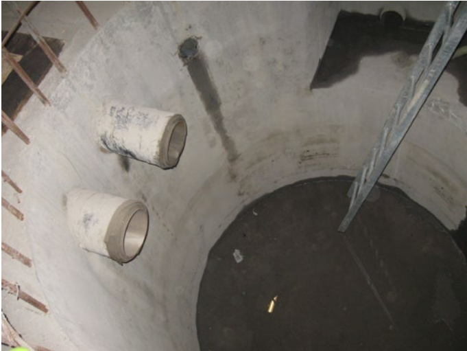
Water ingress into exiting concrete pump station
