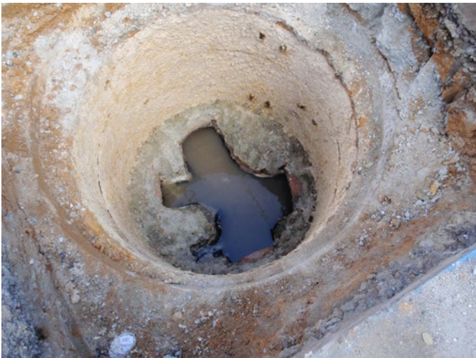
H 2 S attack to concrete manhole
